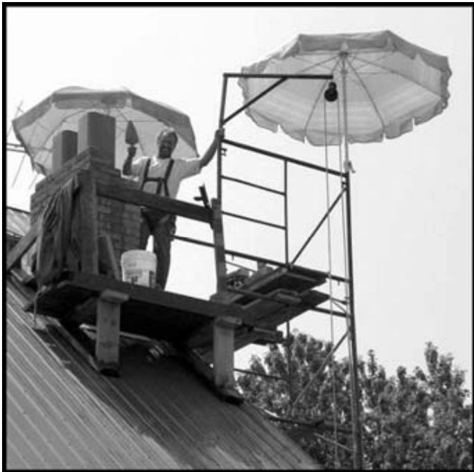
WITH TWO UMBRELLAS PROTECTING HIM FROM THE SUN AND LOOKING VERY MUCH LIKE A SCENE FROM THE MOVIE "MARY POPPINS", JIM VANALSTYNE BUILDS A NEW CHIMNEY ON THIS NORTH SHORE HOME IN THE HAMLET OF EMERALD.
